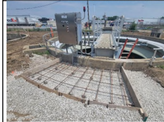
Equipment rack / Control panel installation – CLARI #3
